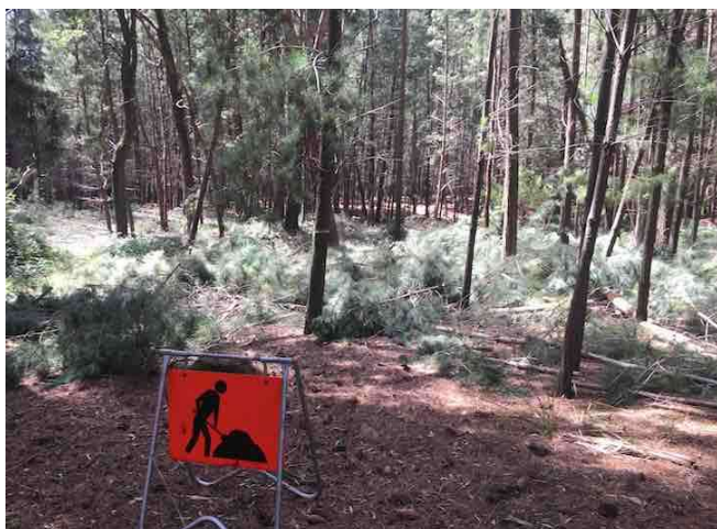
Contracted pine tree removal underway adjacent to the creek. Image 24 th January 2024
