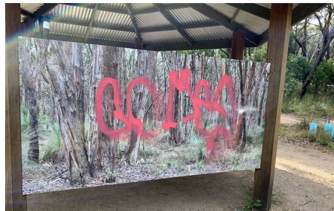
Vandalism at the Dementia Trail Rotunda. Image 21 st January 2024.
