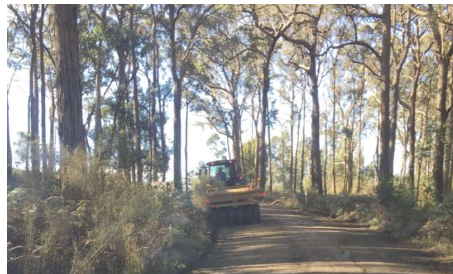
CoB roller on the job, southern side of the Lookout. 2 nd August 2023
