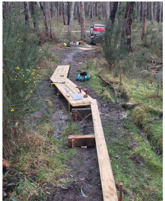
New board walk over a boggy area south of Grasstree Creek on the Cherry Ballart trail. Image 27 th June 2023
