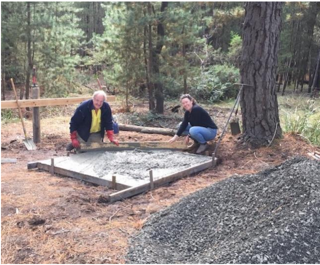
Bob and Hayley smoothing off the table's concrete base. Image: April 19 th 2023.
