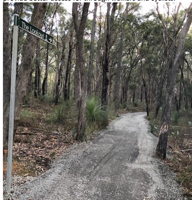
Refurbishment Works underway on the trail. Image May 5 th 2022. Image courtesy of Bill.
