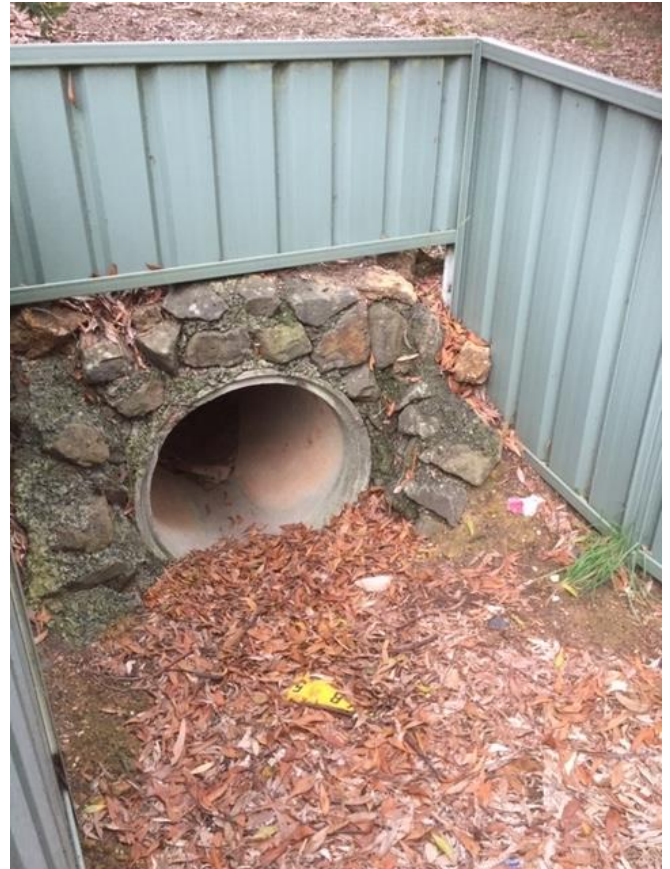
1) The southern entrance of the 50 m long tunnel under the Service Rd and westbound Ballarat turn off dual lane. Image 25 July 2021
