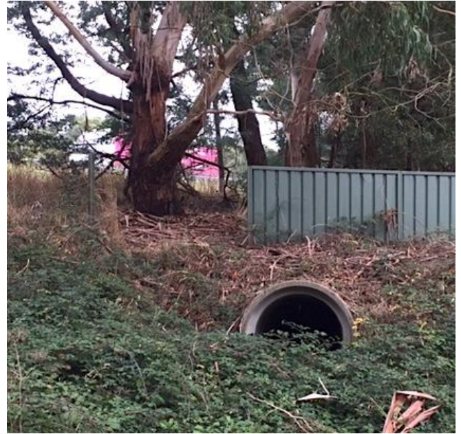
5) Outlet on the North side of the Western Highway with missing fence panels. April 29 th 2022
