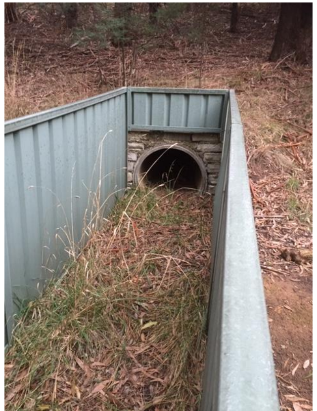
2) 50m Koala tunnel under Eastbound dual lane Ballarat turn off Rd. Image 25 July 2021
