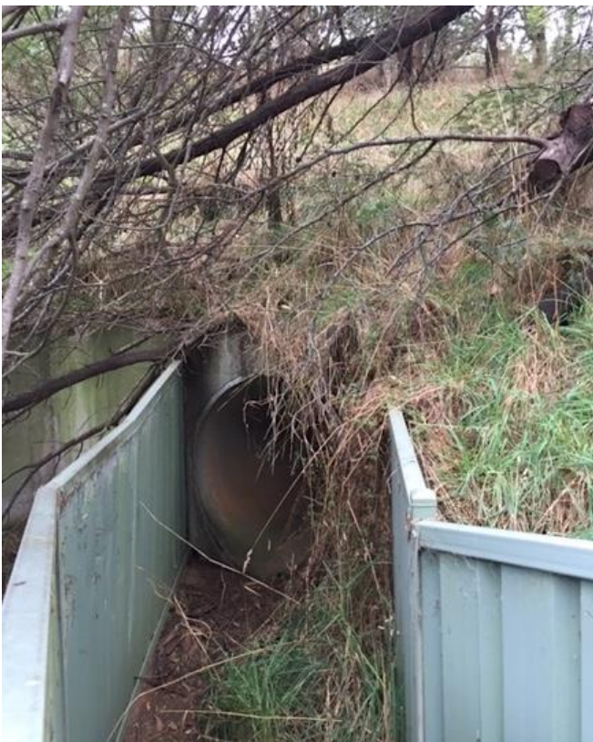
4) South entrance to 100m long tunnel under the Western Highway. April 29 th 2022.
