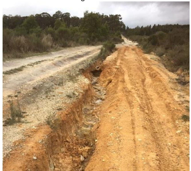
Damaged gully on Baileys Rd. July 22 nd 202
