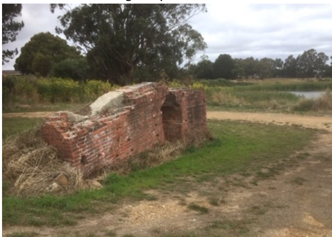
Image: Are these abutments the foundations of Pearces Quartz Mill? January 18 th 2021
